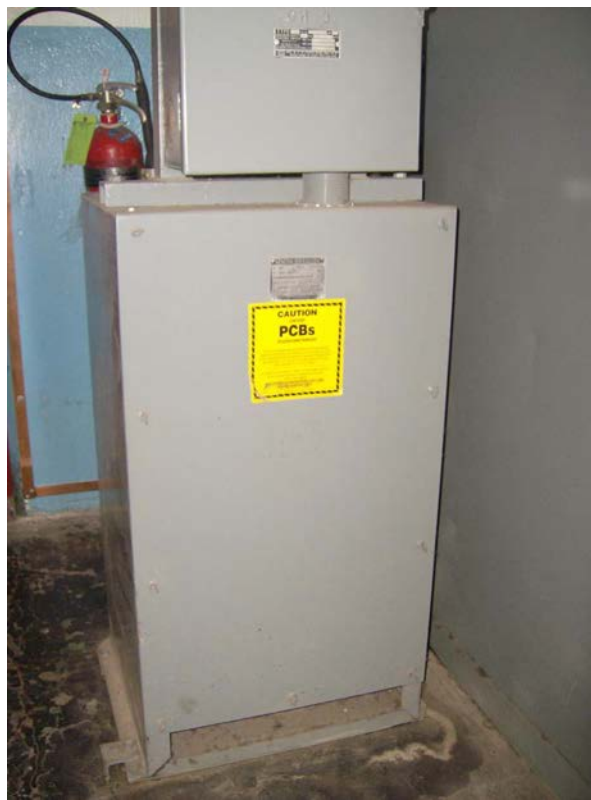
Image 27: PCB-electrical equipment located in existing substations
