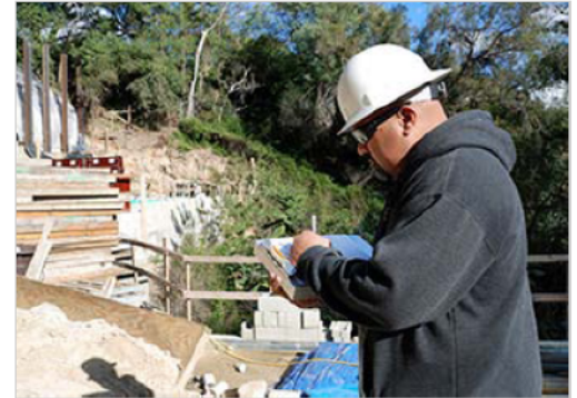
Construction inspectors ensure that building codes are met through all phases of construction.
